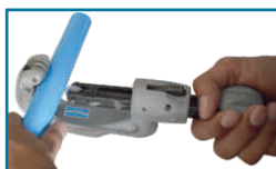
Step 1 : Cutting the Tubes
